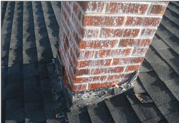
Brick and mortar decay
